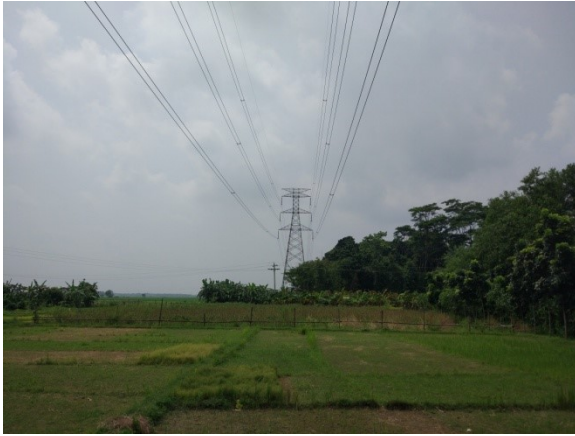
Existing 132kv Electric Transmission Line
