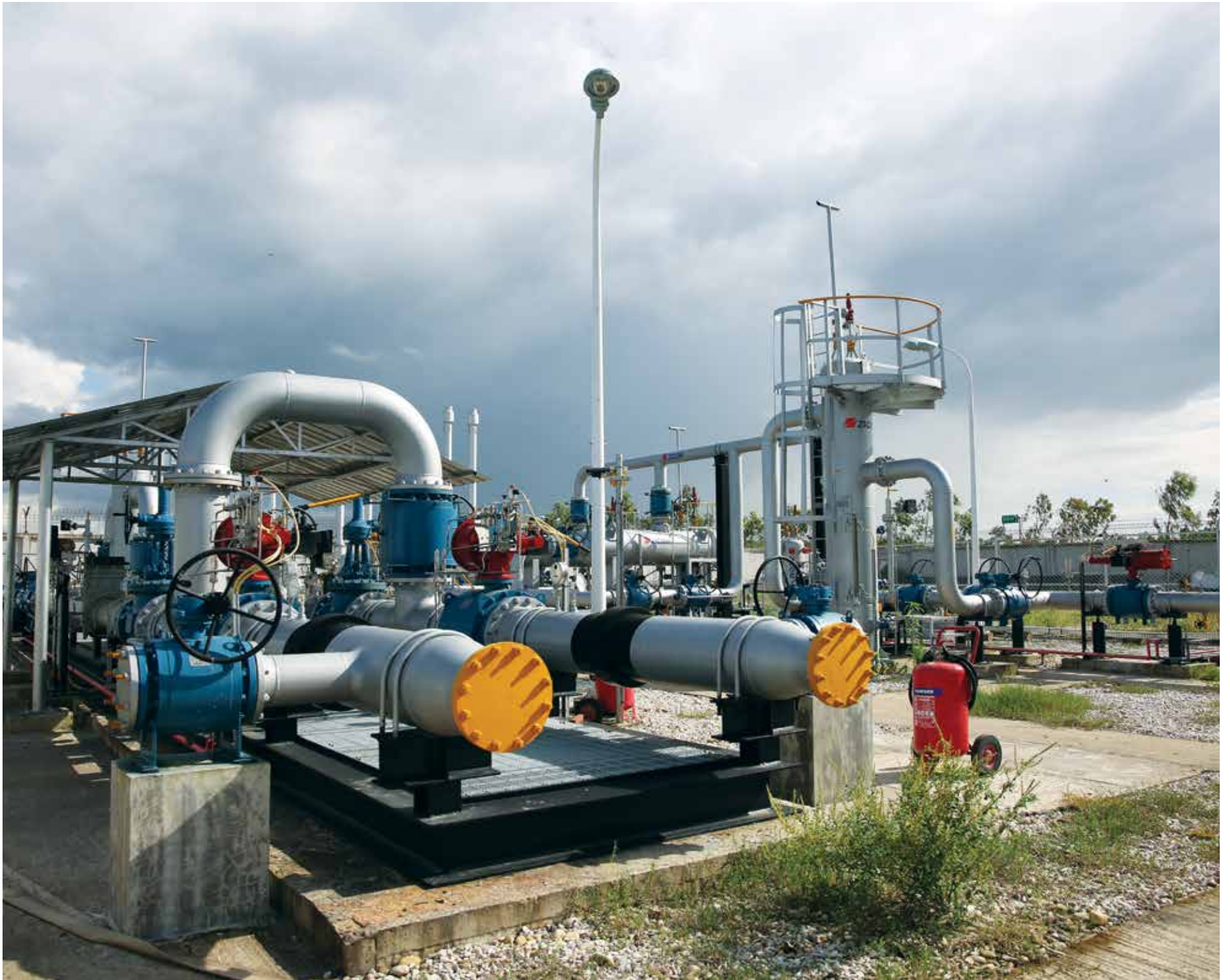
Gas network at Bangabandhu Sheikh Mujib Shilpanagar to serve the investors with quality utility services.
