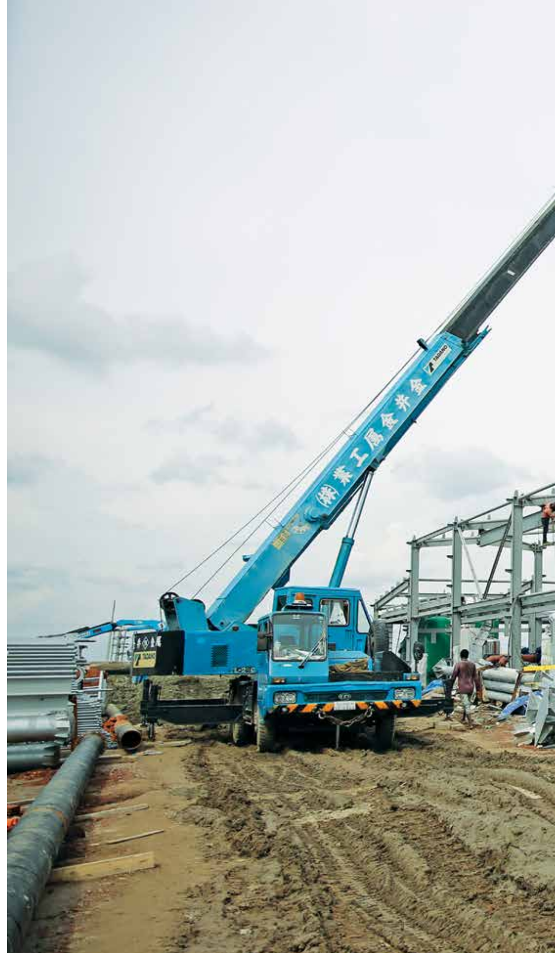
A 150 MW power plant at Bangabandhu Sheikh Mujib Shilpanagar.
