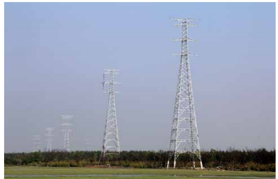
Transmission towers installed by Power Grid Company of Bangladesh (PGCB).
