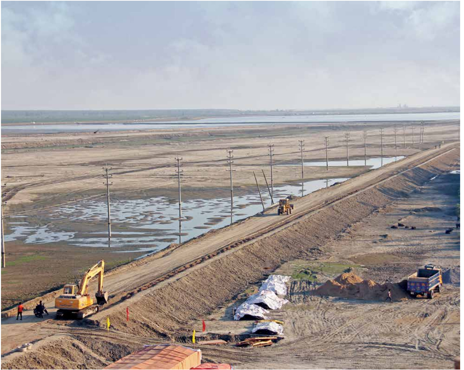
Construction works of a cut-through road, aimed at connecting different zones, is under way.
