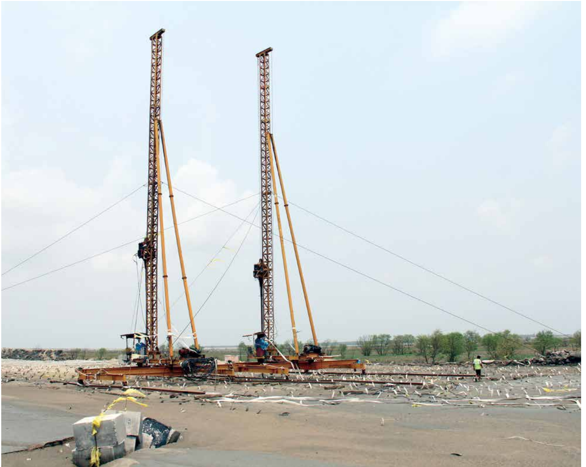
Pre-fabricated vertical drains with pre-loading of soft clay are being used to improve the soft soil.
