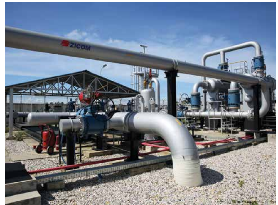
Gas supply facility set up by Karnaphuli Gas Distribution Company Limited (KGDCL).
