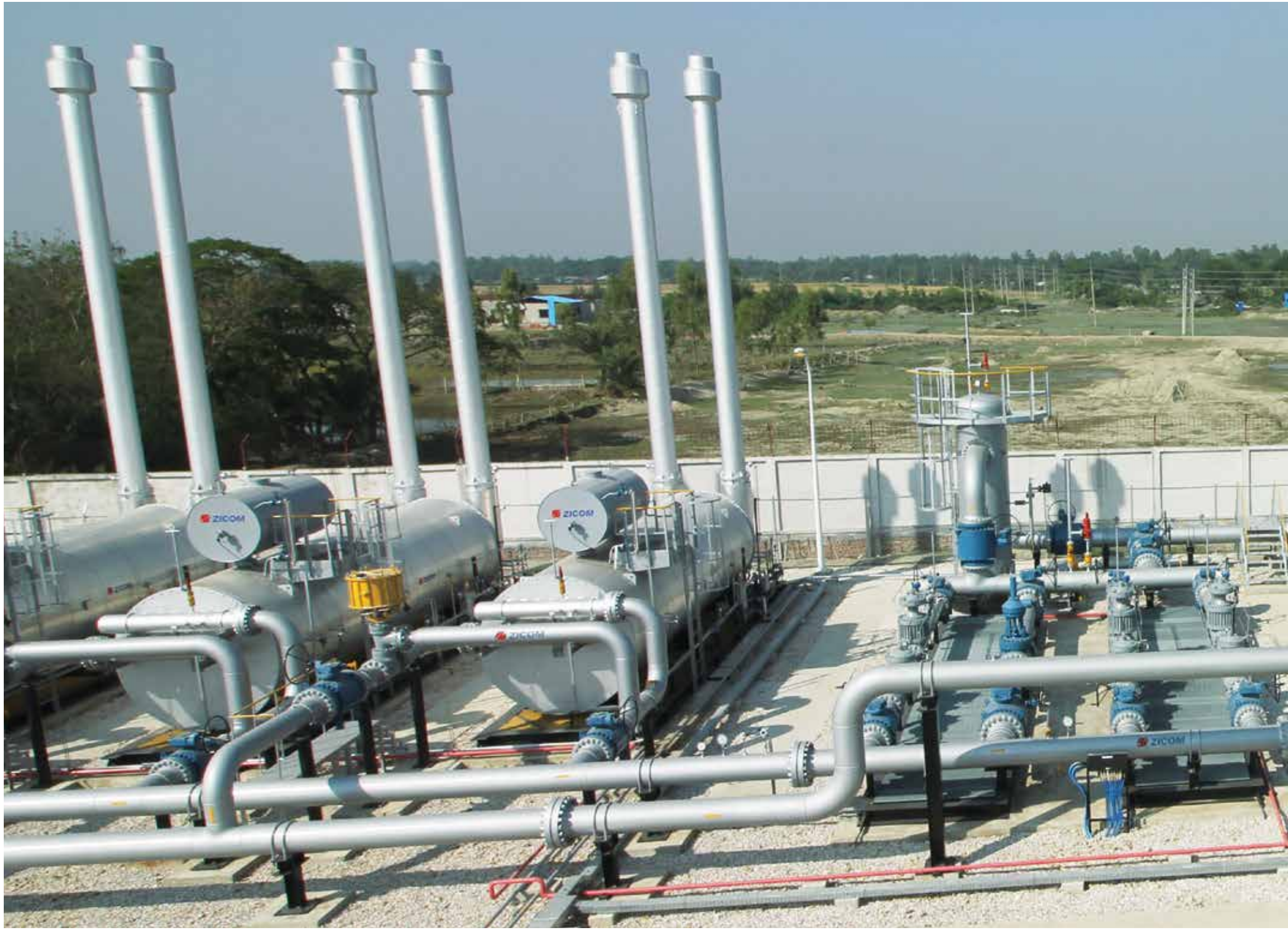
The Karnaphuli Gas Distribution Company Ltd (KGDCL) has upgraded its existing gas distribution network from 350 mmcf/d to 500 mmcf/d to facilitate adequate gas supply to industrial customers.
