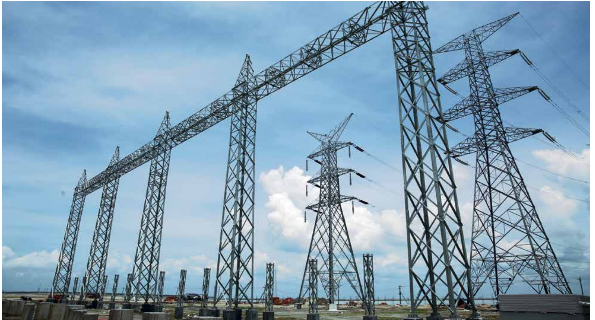
230 KVA Grid Substation / Transmission line in the industrial city.
