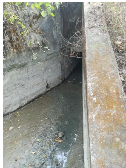
Figure 2.7: 1 vent regulator of Golla Donakhali khal
