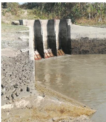
Figure 2.2: 3 vent regulator on Domkhali khal
