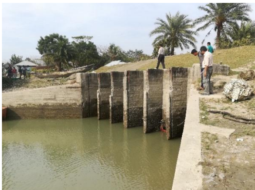
Figure 2.4: 6 vent regulator of Shaherkhali khal
