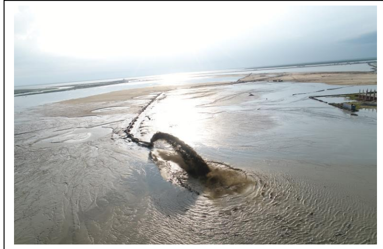
Photo-9-3: Pipeline for transporting dredged material
