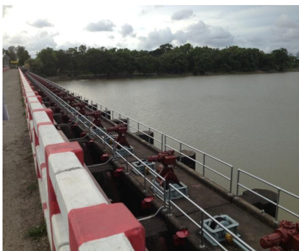
Sluice gate (Regulator) at intersection of Feni River and Muhuri Project Embankment at north of the project site with upstream view of Feni River to the right.
