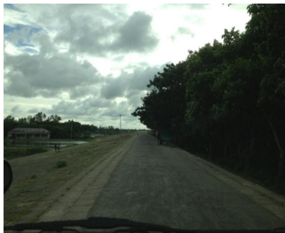
View of Muhuri Project Embankment with very mild side slope to the Bay side near the project starting point. Project site (northern part) is seen to the left.
