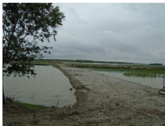
Access Road for Mirsarai - 2A EZ at main access road for both Mirsarai 1 and Mirsarai 2 with view of Mirsarai 1 to the right
