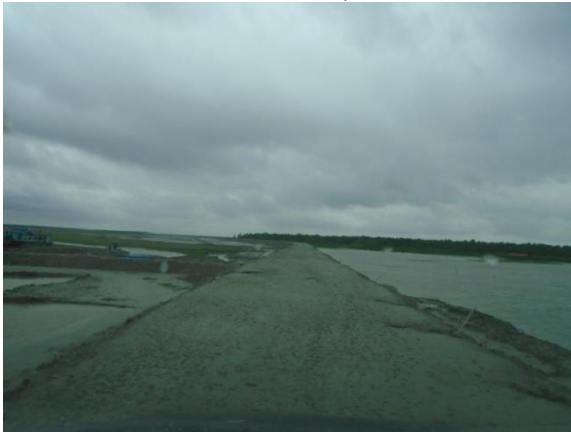
View of Access road for Mirsarai-2B. This is also north side embankment of Mirsarai 1 EZ.
