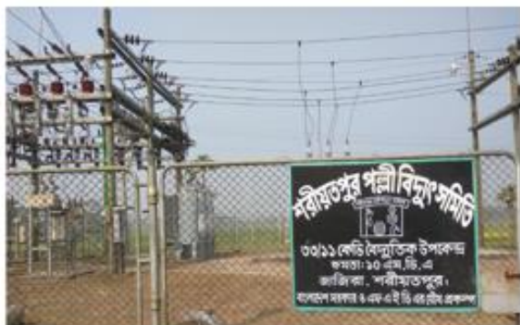
Operational substation towards south of EZ site
