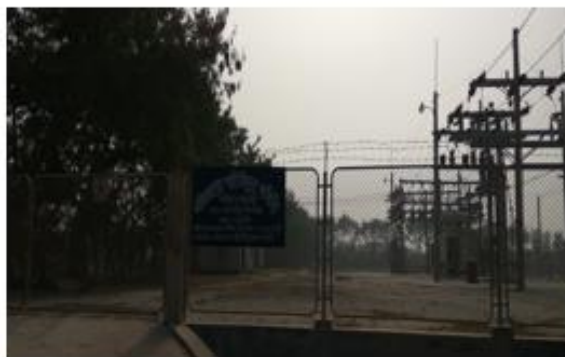
Operational substation on north of EZ site
