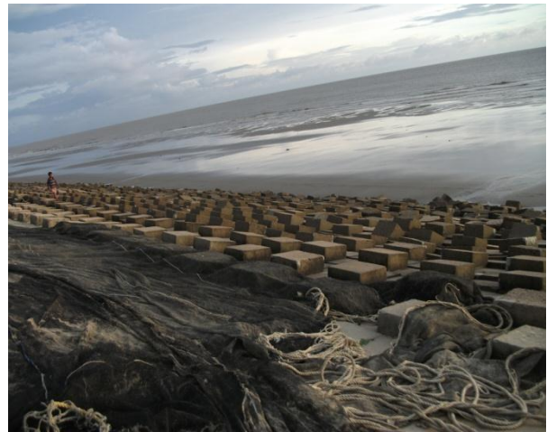
Photograph shows dike with displaced concrete blocks and washed road on top.
