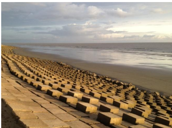
View of side slope protection work of Embankment with displaced concrete blocks along the toe line.
