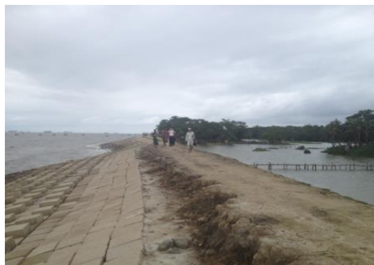
Photo of dike with washed road on top (LHS –Bay of Bengal; RHS -Site)
