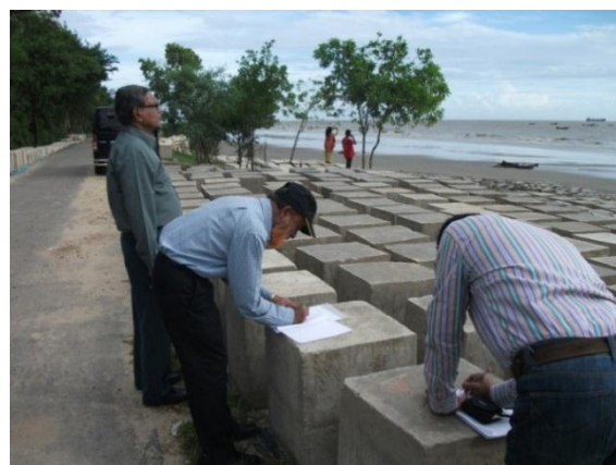
View of BWDB Embankment towards project site near Parky Beach Bazar. Paved road top apparently in good condition. Concrete blocks are ready to be used for side slope protection of Embankment.
