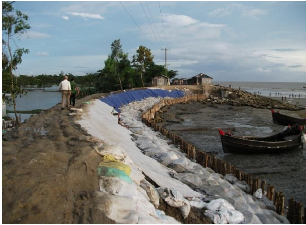
View of Embankment in very poor condition with water body at project site to the left.
