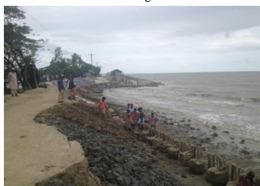
Landslide mitigation work going on at site (facing the Bay of Bengal)
