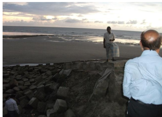
View of Embankment side slope failure.
