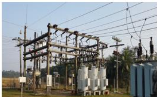
Currently operational substation at Dakbangla
