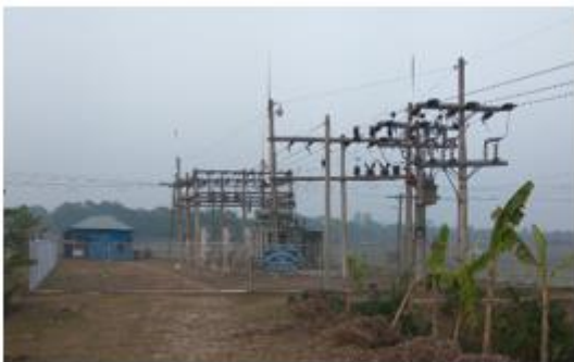
Substation towards south east of Gopalganj site
