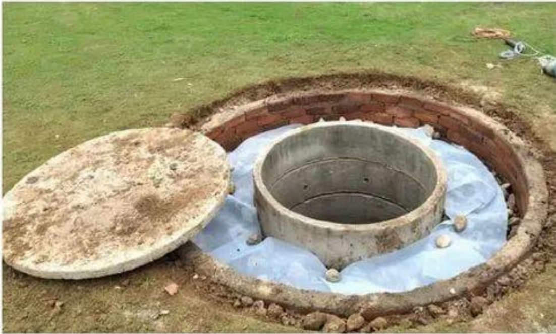
Figure 4.20: Recharge pit of Rainwater Harvesting System (RHS)
